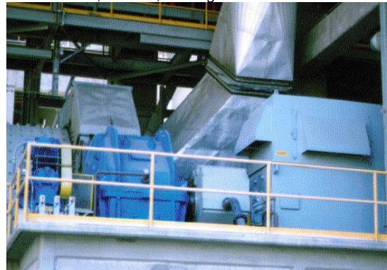
3880kW, 4.16kV, 900rpm synchronous motor Fluid coupling, ball mill drive
