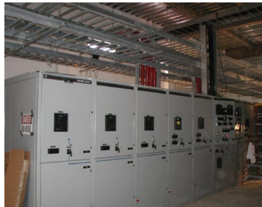
15kV Vacuum metal clad switchgear
