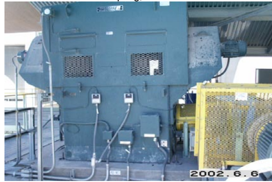
1100 kW, 1800rpm, 4.16 kV, kiln drive motor & VFD Please visit our WEBSITE or contact us at:
