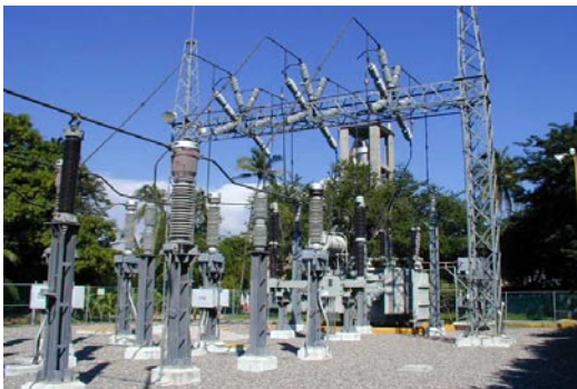
138kV, 3ph, 60 Hz incoming substation
