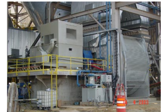
8300hp, 13.8kV, synch Motor-Fluid coupling
