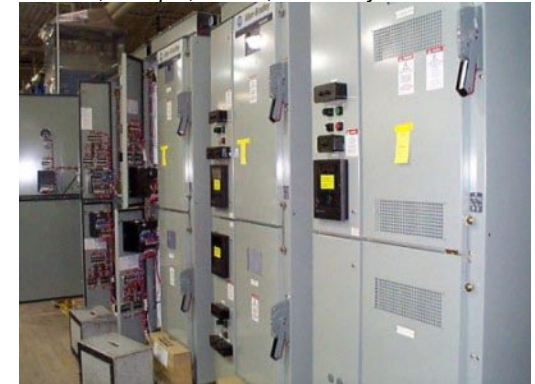
5kV VFD incoming and bypass switchgear
