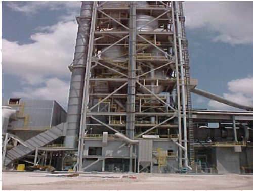
2200 TPD steel preheater tower
