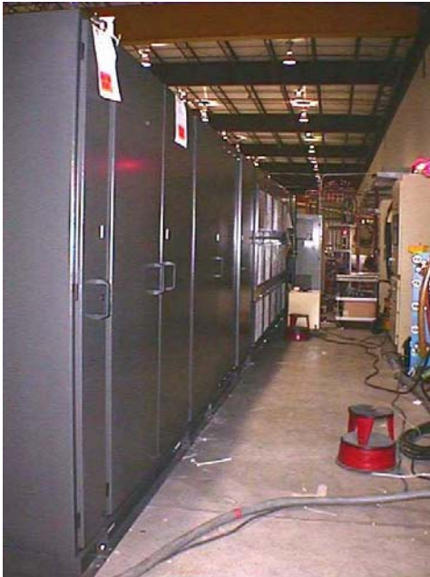
Figure 3 – 2000kW VFD, 6000V/50Hz, on the test bay
